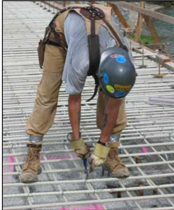
Figure 11.8: A construction worker stands on glass FRP bars while tying them together (courtesy Vector Construction Group).
