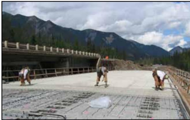
Figure 11.3: Placement of glass FRP bars in a bridge deck (courtesy Vector Construction Group).
