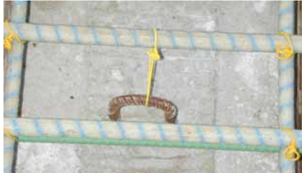
Figure 11.6: Glass FRP rebar tied down with plastic-coated steel ties (courtesy Vector Construction Group).
