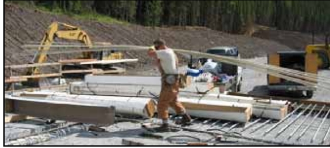
Figure 11.2: Lightweight bundles of FRP bars are easily moved on site (courtesy Vector Construction Group).
