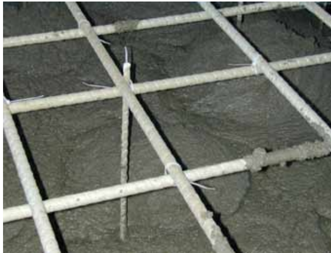
Figure 11.4: Glass FRP rebar tied with nylon zip-ties and glass FRP chairs to eliminate all corrosion (courtesy Vector Construction Group).
