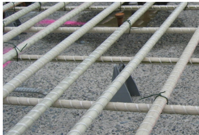
Figure 11.5: Glass FRP rebar tied with standard steel ties and using plastic chairs (courtesy Vector Construction Group).
